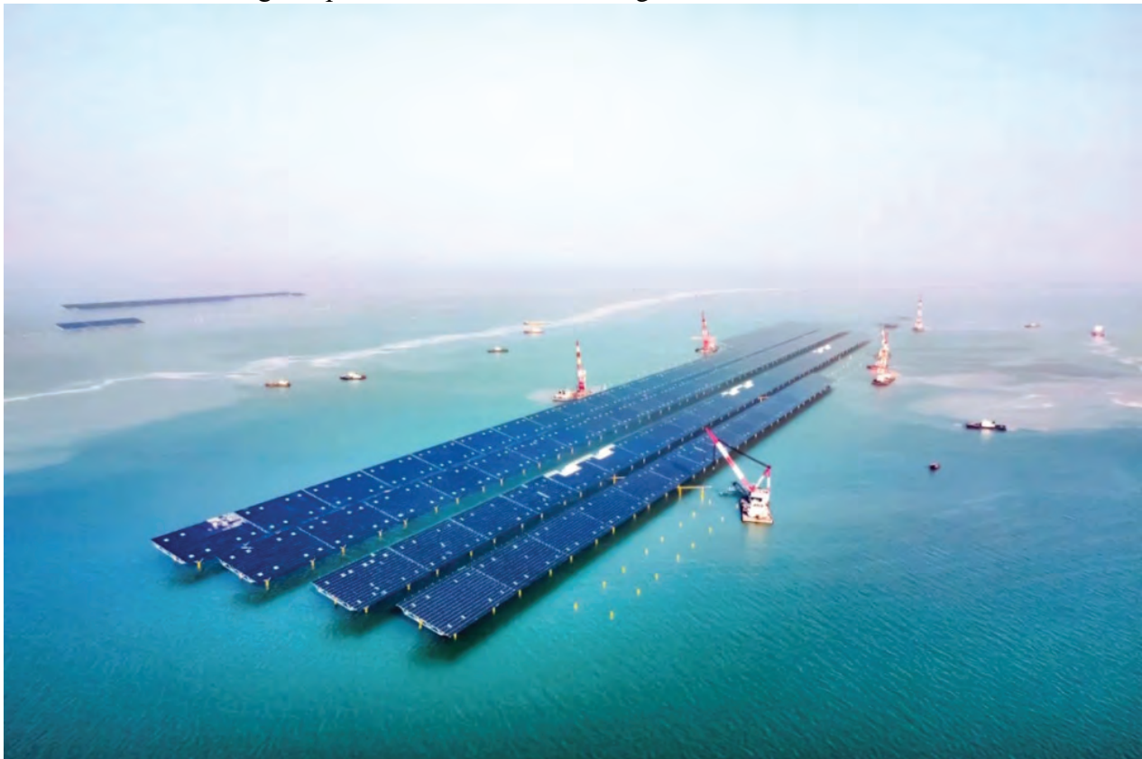
Aerial view of Guohua Energy Investment's 1-gigawatt offshore PV project in Kenli, Shandong
